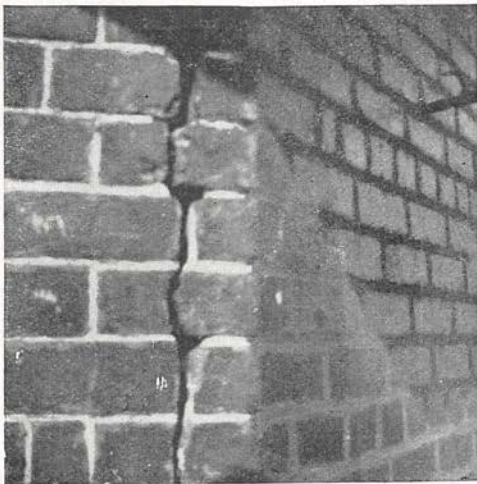
UGLY CRACKS EXTENDED DOWN THE SIDES FOR 150 FEET.
