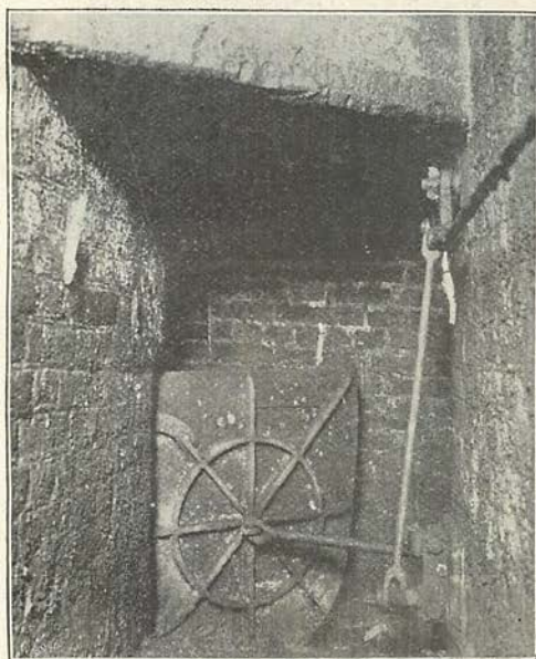
FLUSHING GATE OF ORDINARY SEWER.
