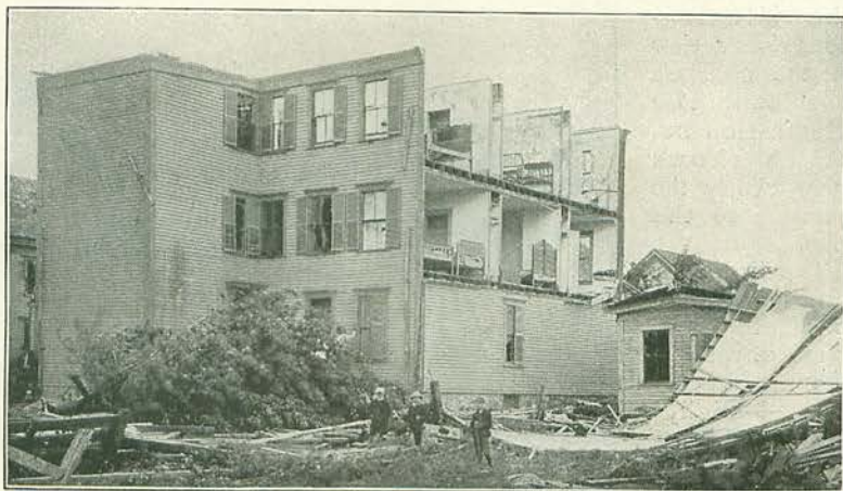
ROOF AND SIDE OF HOUSE CARRIED AWAY AT LAWRENCE, MASS. From a Photograph. Lent by Royal Meteorological Society.
