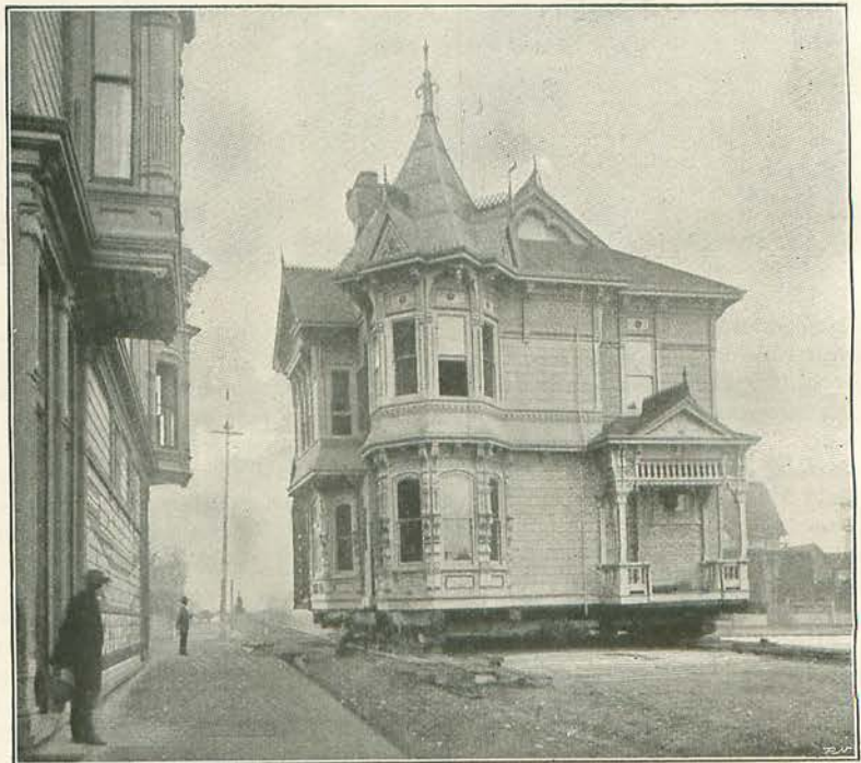
THE HOUSE BEING PULLED ON ROLLERS TO ITS DESTINATION IN EUREKA, CAL.
