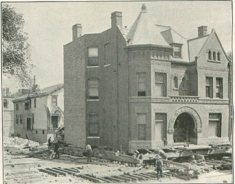
DOUBLE BRICK RESIDENCE IN CHICAGO BEING TURNED FROM NORTH TO SOUTH FRONT, WITH PEOPLE IN OCCUPATION. [E. L. Clements, Chicago.] From a Photo. by]
