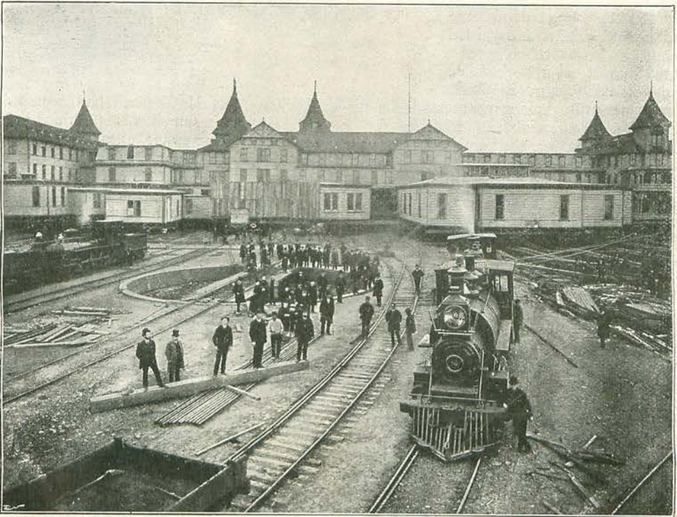
SIX LOCOMOTIVES PULLING THE BRIGHTON BEACH HOTEL BACK FROM THE OCEAN, APRIL 3RD, 1888—THE ENTIRE BUILDING RESTING ON 112 FLAT TRUCKS. [Photograph.]
