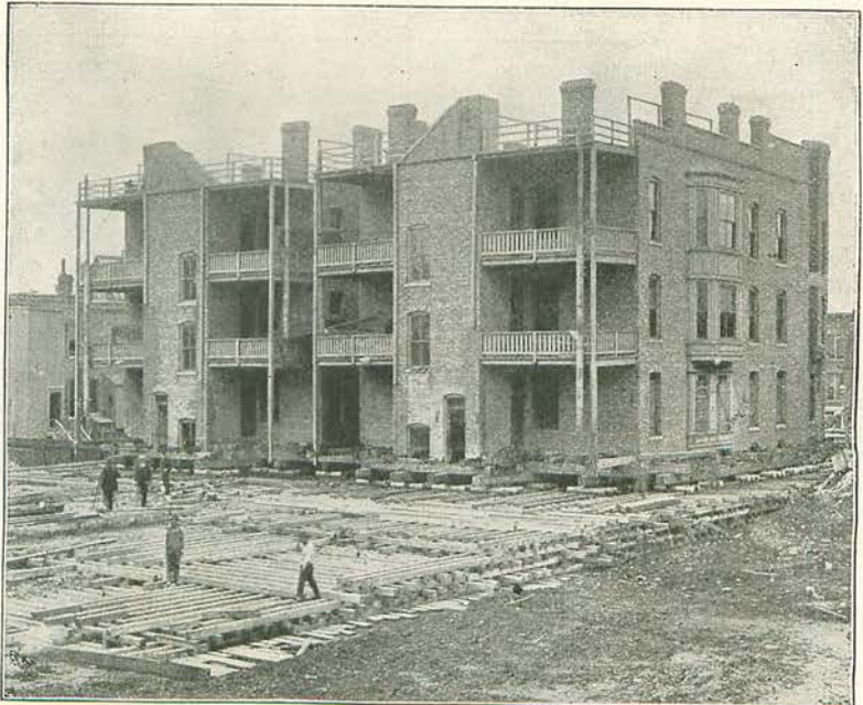
APARTMENT BUILDING OF 8,000 TONS IN CHICAGO BEING MOVED TO MAKE WAY FOR AN ELEVATED RAILWAY.
