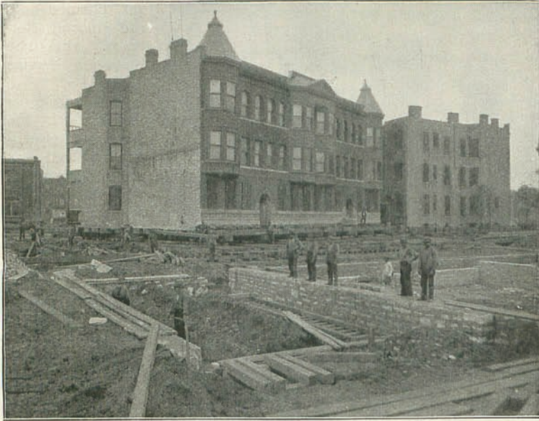
MAKING WAY FOR THE METROPOLITAN ELEVATED RAILWAY IN CHICAGO—NEW FOUNDATIONS IN FOREGROUND. [E. L. Clements, Chicago.] From a Photo. by]
