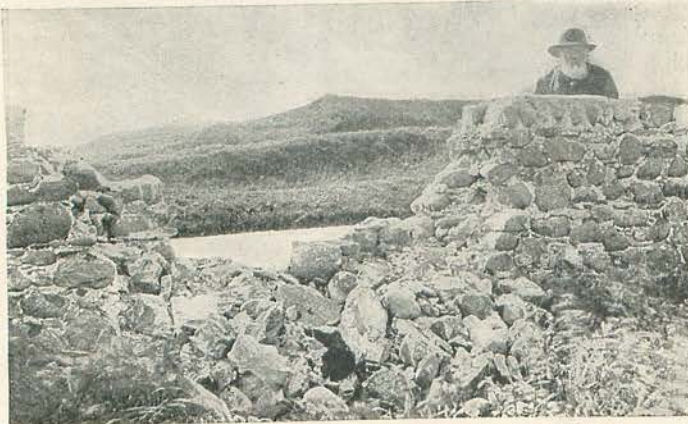
19.—STONE WALL BROKEN BY LIGHTNING AT ALLONBY, CUMBERLAND. From a Photo. lent by G. J. Symons, Esq., F.R.S.
