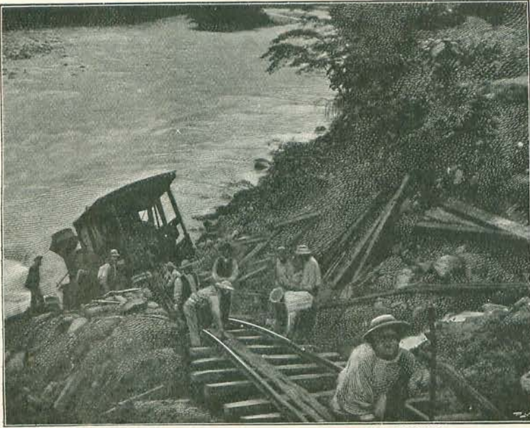
5.—REPAIRING DAMAGE BY FLOOD ON THE COSTA RICA RAILWAY. From a Photograph.
